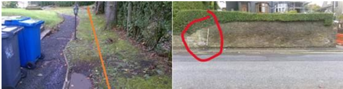
Image 2 - Illustrates my main gas line entering the external wall onto the property and past the tree roots to the dwelling which has been replaced on Dec 28 th 2021, due to a gas leak at the entry of the property. I was advised by my gas company that the soil and roots pushing towards the main gas pipe have caused this.
