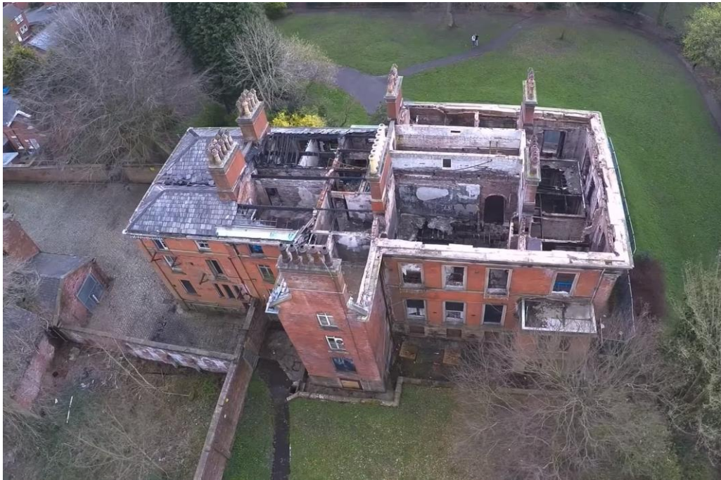
Figure Four – Drone Photo Showing Derelict Condition of the Lodge
